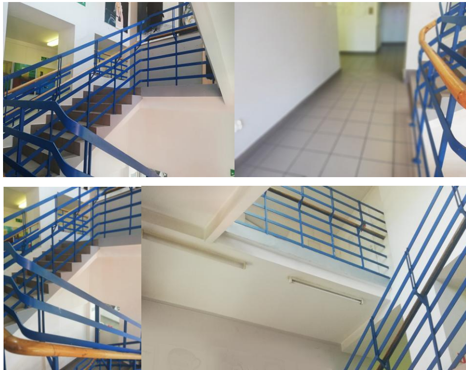
An example of a place presented in the photo, the 4 th floor of the building of the Faculty of Visual Arts, the author's original photo, 2017.
